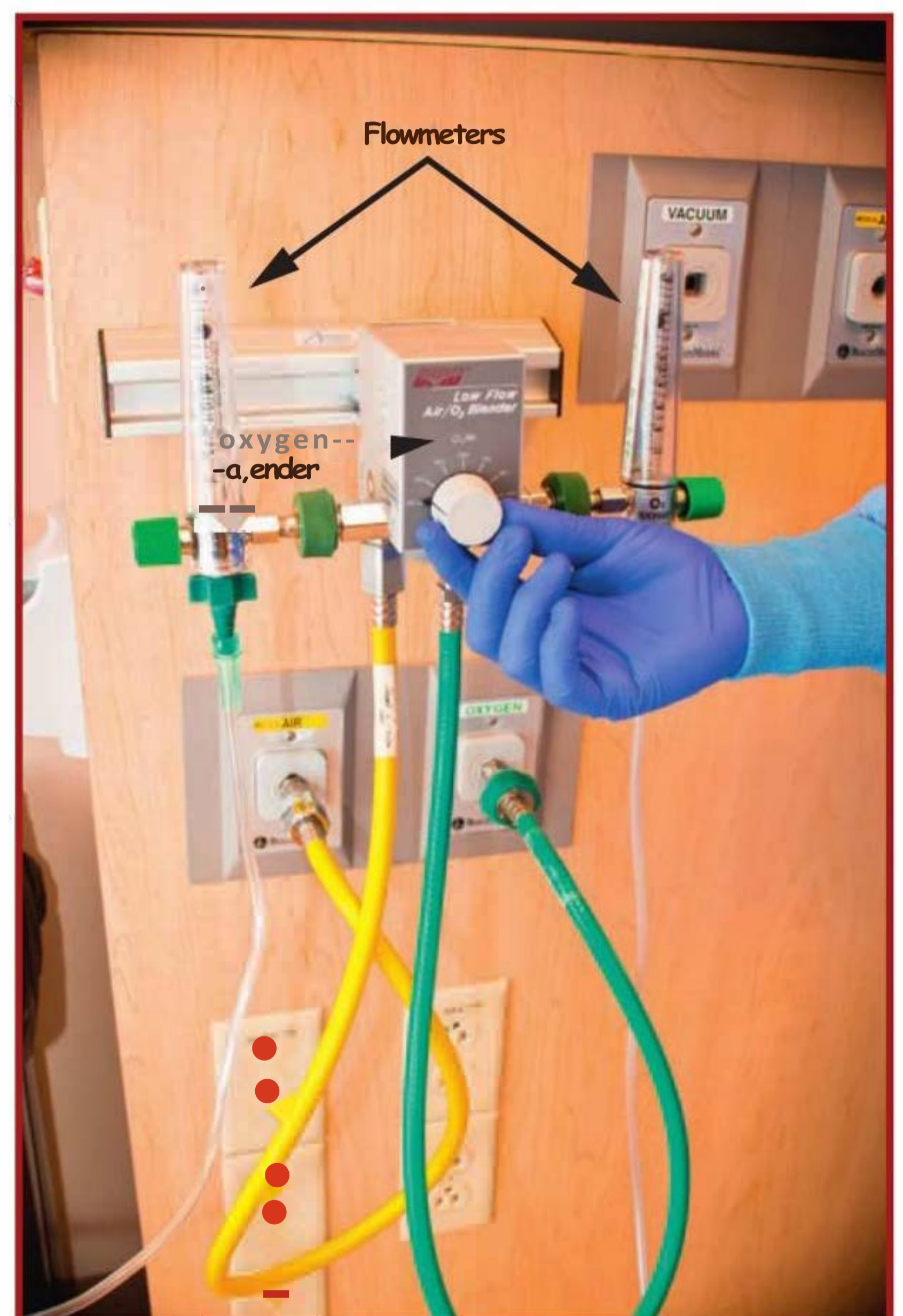
Figure 3.17. Adjust the concentration and flow of oxygen with compressed air (inflow from yellow hose), compressed oxygen (inflow from green hose), an oxygen blender, and a flowmeter. The image shows 2 flowmeters attached to the oxygen blender. Your system may only have 1 flowmeter.
