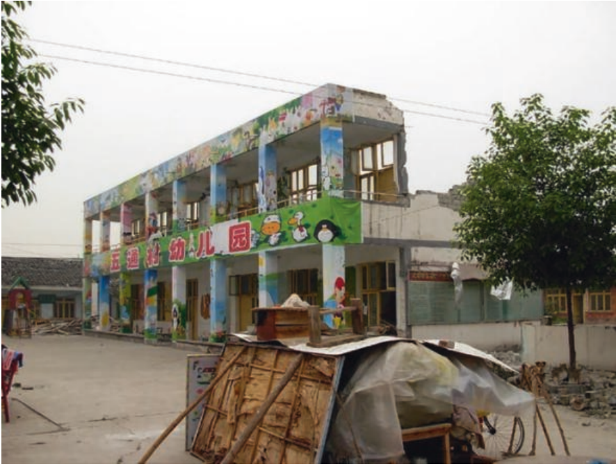
Fig. 8.3 This kindergarten was one of the many schools badly damaged, 2008 Sichuan earthquake. (Courtesy of Wikimedia Commons)
